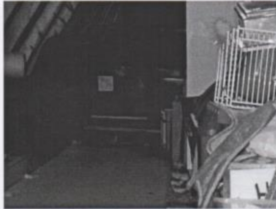
Incorrectly supported tanks
