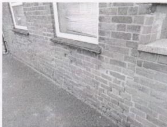
Spalling to face brickwork
