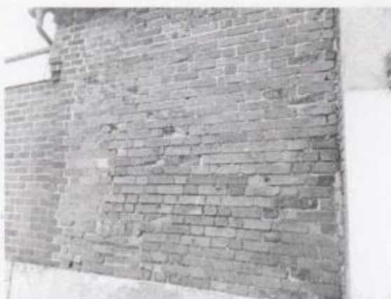
Delaminated and refaced bricks.
